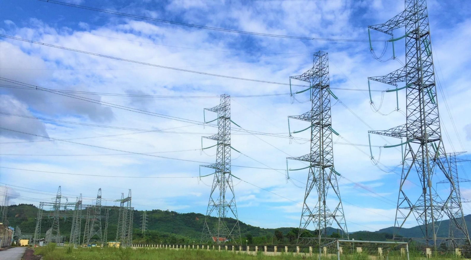
Note: 500kV transmission line, in the 500 kV Quảng Ninh substation area. Copyright @VIET
